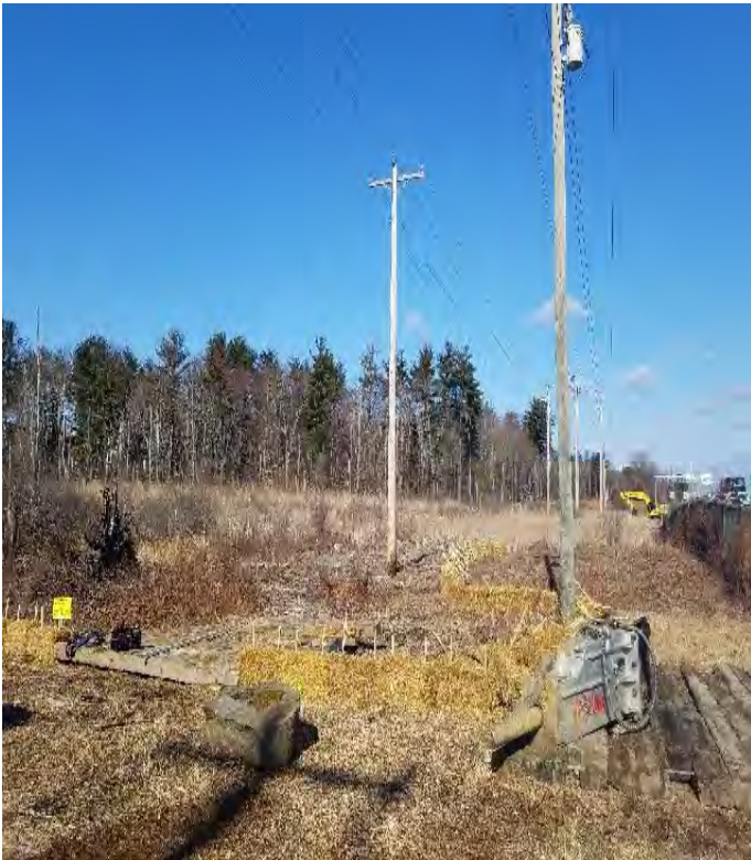
Fig 19: Prepping to excavate foundation for Str. 129. BMPs installed Between work area and wetland NW1. Viewing west. (03-04-20).
