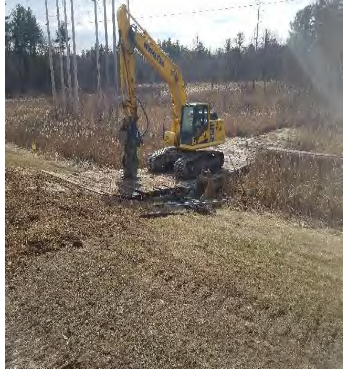
Fig 10: Crew beginning to build matted work pad for Str. 128, in wetland NW1. Viewing south. (03-02-20).
