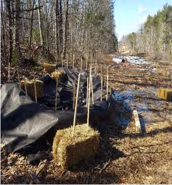
Fig 17: Dewatering basin built across Timber Brook Lane to dewater Str. 63. Viewing south. (03-04-20).
