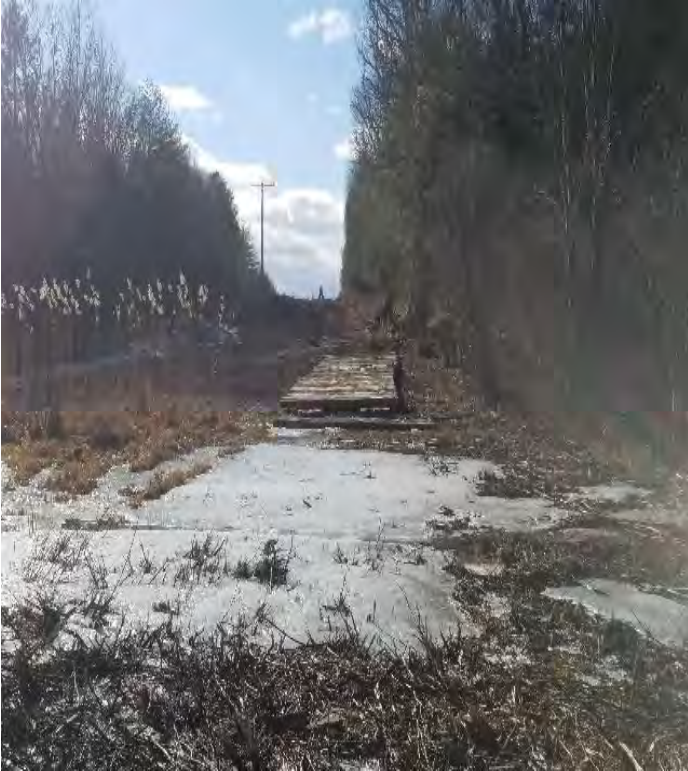
Fig 1: Building access road from Str. 74 to Str. 75. About to mat through wetland DW21. Viewing west. (02-28-20).
